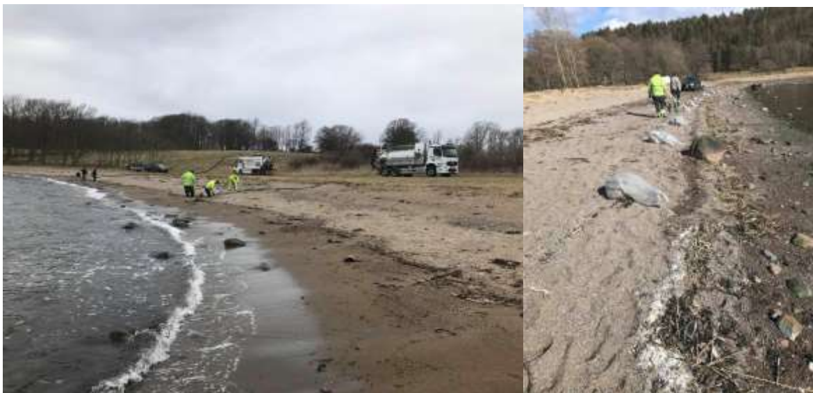
Figure 13. Reier beach in Moss municipality. Here a suction vehicle is being used.
